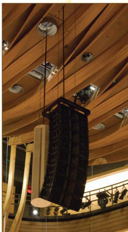
TOP: FIBRE-ORIENTED PATCHBAY. IN THE FUTURE, XLR CONNECTORS WILL BE REPLACED BY FIBRE OR CAT-5 CONNECTORS & PORTABLE RACKS WITH PREAMPS THAT MOVE TO WHEREVER THE INPUTS ARE NEEDED & PLUG INTO A FIBRE PORT. RIGHT: CENTRE CLUSTER OF JBL POP ARRAY, WITH TRAP DOOR ABOVE.
