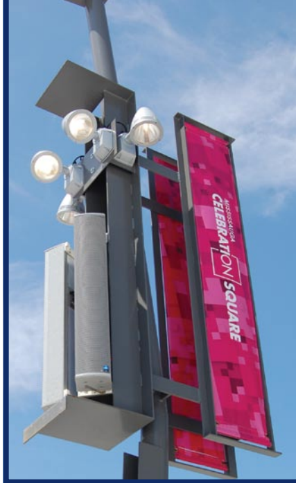
FAR LEFT: Mobile production cart with APB ProRack mixer hooked into network at amphitheatre position. LEFT: Renkus-Heinz ICONYX IC Live arrays mounted onto light fixtures. BOTTOM LEFT: DiGiCo SD8 at FOH, connected to fibre network via access node.
